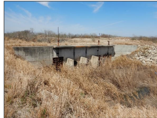
Photograph 29 – View looking northeast at the control structure that controls water flow from the existing Raymondville Drain to La Sal Vieja.
